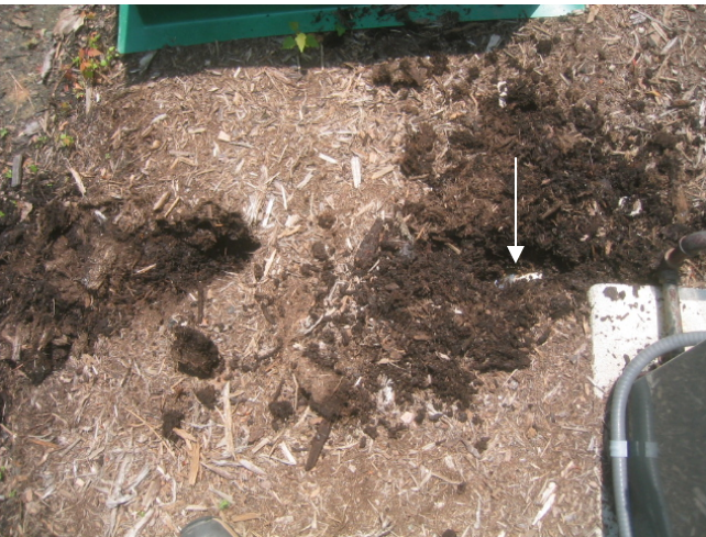
Gas pack air conditioning condensate drainpipe does not currently drain to daylight
