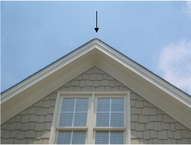
Garage gable roof end ridge cap shingle is damaged
