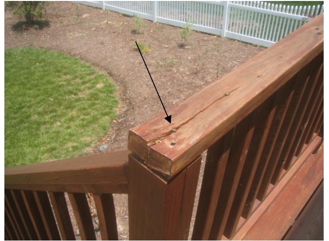
Rear deck rear right handrail upper rail is split and warped
