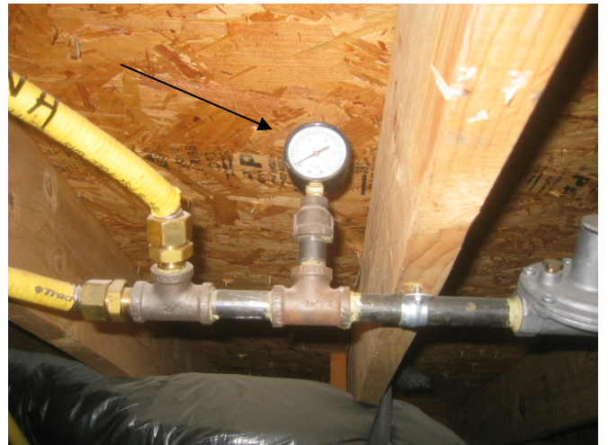
Attic natural gas supply manifold has a temporary type pressure gauge still installed
